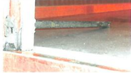
Door securing 'stay bar, looking through grain hatch
